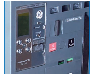
Trip unit and all indicators are visible through the door
