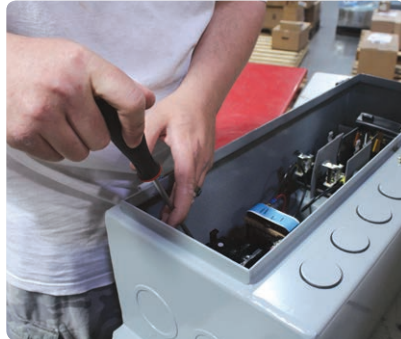
2 Combination Enclosed Starter- Being modified
