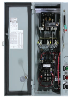
3 Combination Enclosed Starter- Modified and ready to ship
